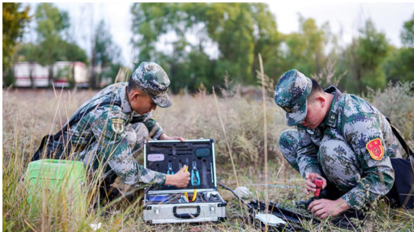
Members of a PLASSF unit undertake field repairs on a fiber-optic cable 255
